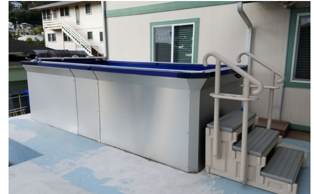
Aboveground Outdoor Installation
